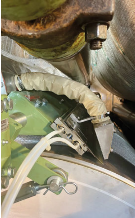
▲Dust removal system.
